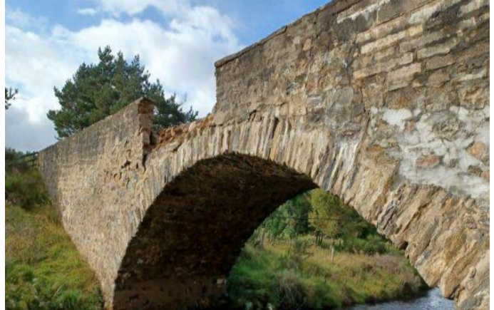
A939 Dava bridge was stuck by a car during September 2023 leading to significant damage and closure of the bridge. (photo Highland Council)
