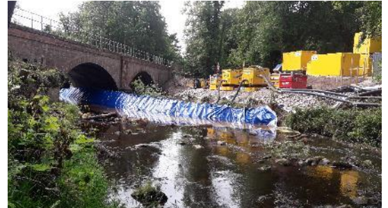
The Brodie Railway bridge repair required a portadam to be installed and water pumps to dry out the site prior to in river works.
