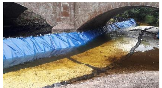
Concrete mattress laid below the bridge to strengthen and stabilize the foundations. Substrate was infilled on top to provide a natural riverbed structure and complete repairs.
