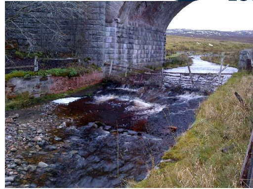
Scour protection under the Dalmagarry rail bridge requiring repair
