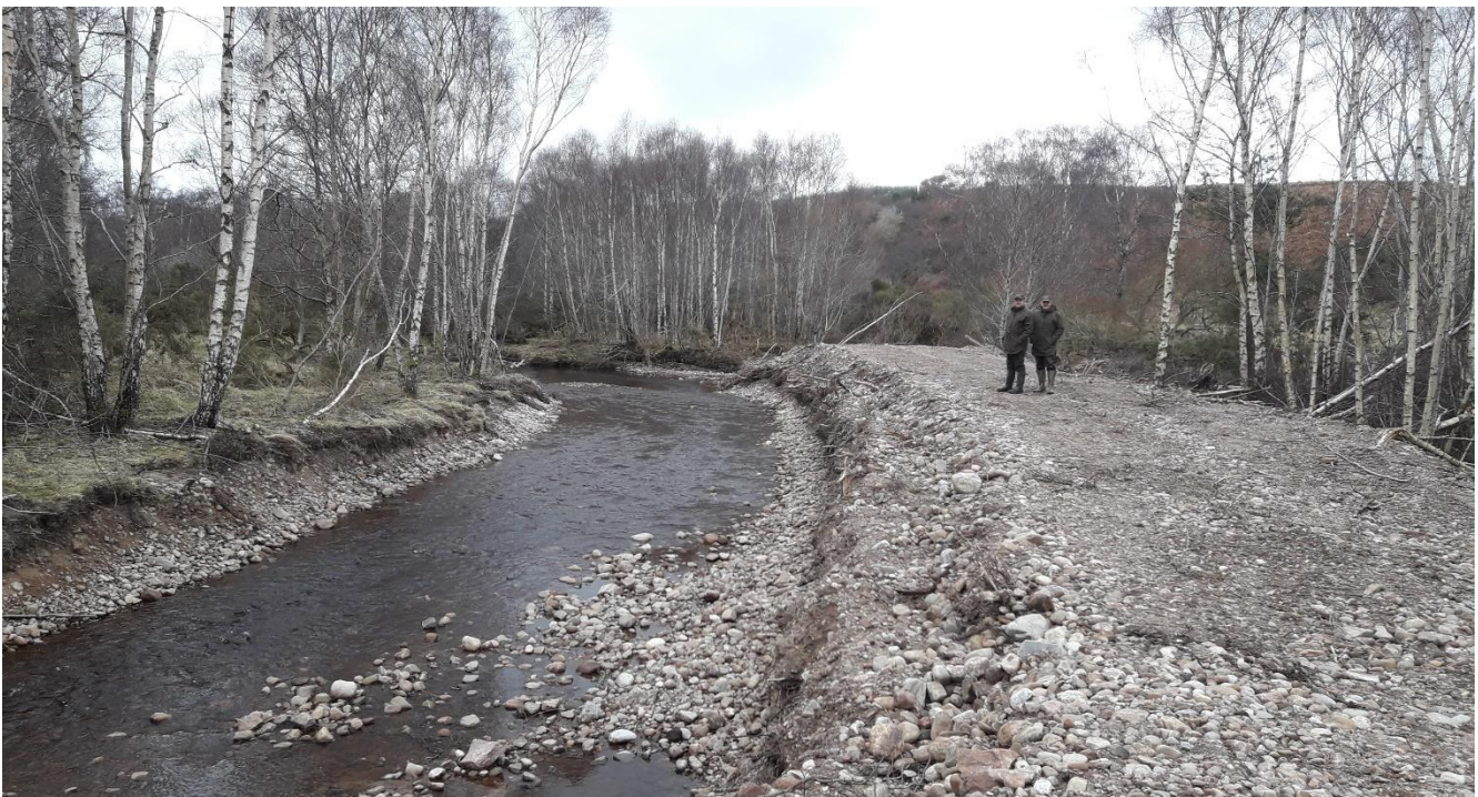
Sean and Ali inspecting re-channeling works at Achavraat on the Muckle Burn, March 2021.
