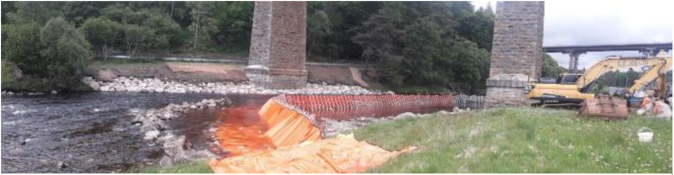
Installing the portadam around the right bank pillar of the Tomatin railway viaduct, June 2020.
