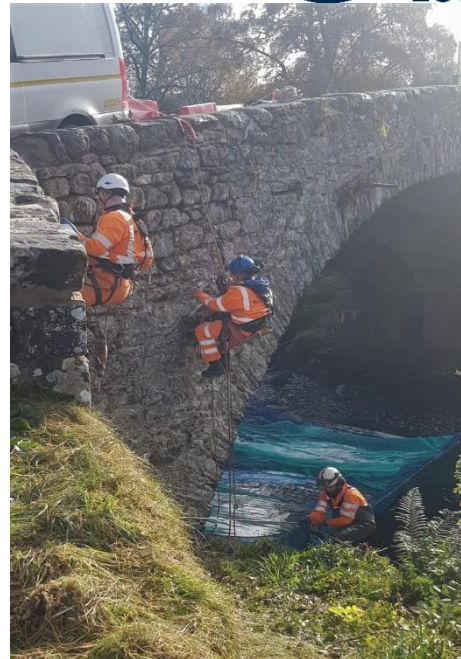
Repair works underway at Bantrack Bridge River Divie Oct 2020. (Photo Sean Maclean)
