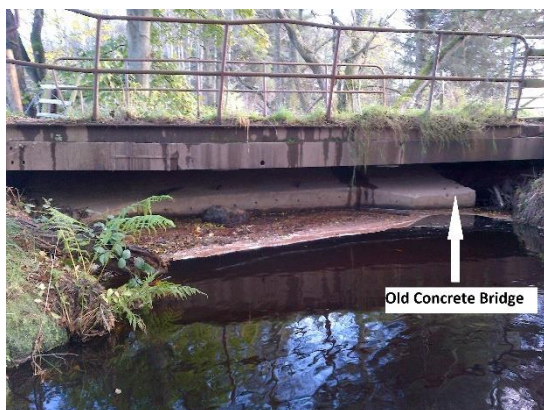
Burnside Bridge on the Black Burn, showing collapse concrete bridge and temporary bridge platform.
